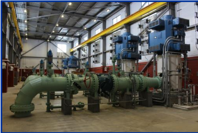
Pumps in the raw water pump station building
