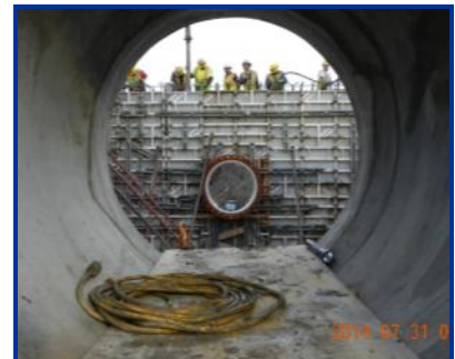
Discharge valve vault at Williams Creek Pump Station
