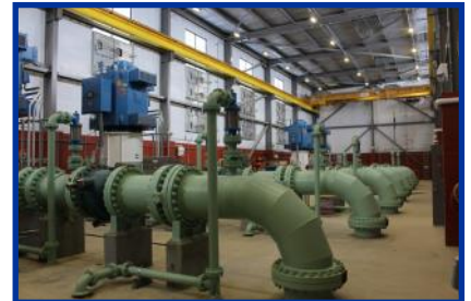
Bradley Pump Station pump room
