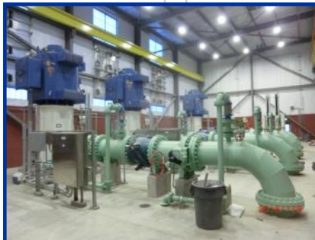
Pump room at Juniper Pump Station
