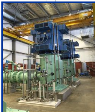
Bradley Pump Station pumps
