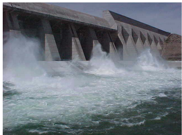
Full releases from Pueblo Dam to the Arkansas River following the completion of SOD work in 2000.
